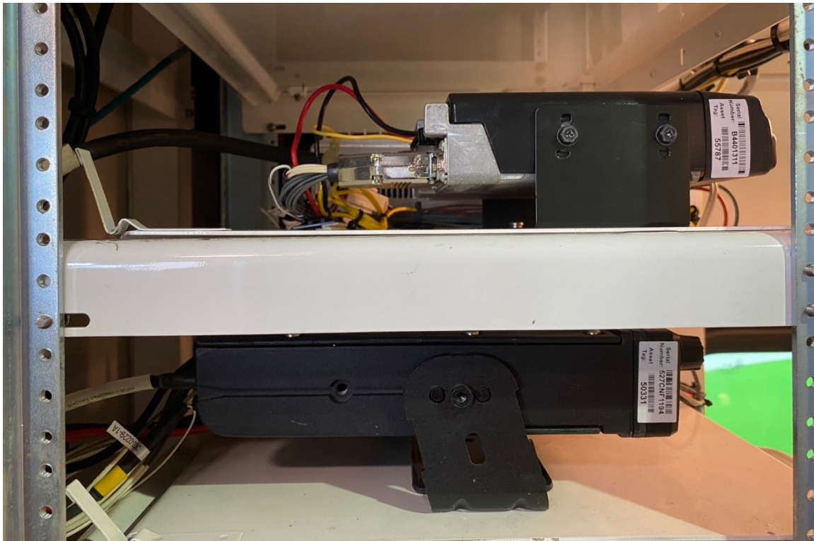
Figure 3: Clearance at the rear of the equipment
