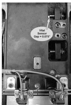
Figure 329(d)(2)-02: Lock Box Sensors
