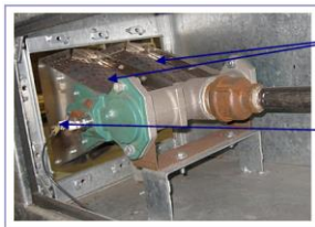
Figure 612(a)-2: The Burner Unit
