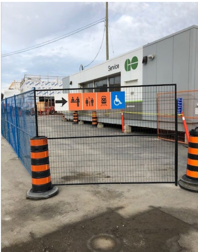
Photo 4: Signage uses current Metrolinx wayfinding design standards and is secured at a logical wayfinding point
